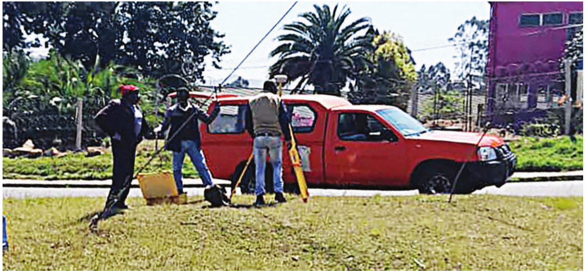
▲ Men from the Municipal City of Mbabane setting up a land surveying machine in Mbabane, Mahlokohla Street.
