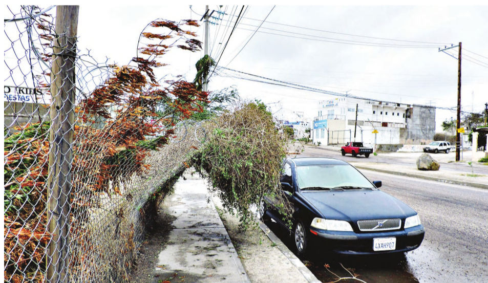
▲ A view of a leaning fence.
