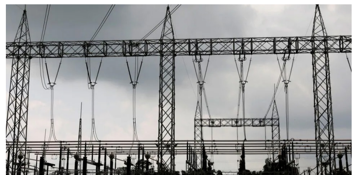
▲ High-tension electrical power lines are seen at the Azura-Edo Independent Power Plant (IPP) on the outskirts of Benin City in Edo state, Nigeria
